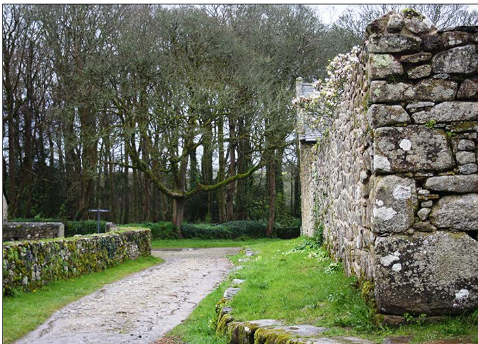
A view down the western side of the King's Garden wall after conservation showing primroses emerging on the raised walkway
